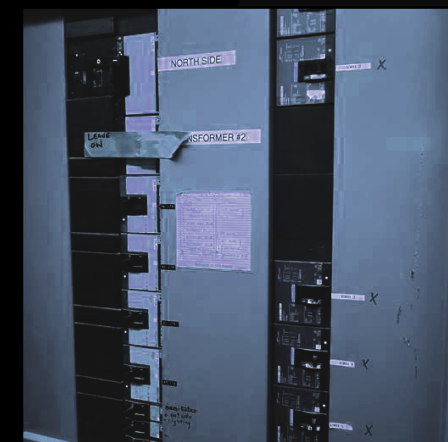
POWER AND CONTROL INFRASTRUCTURE
